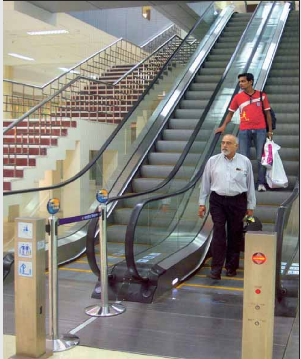
SJEC Johnson Escalators installed at Anna International Airport, Chennai
