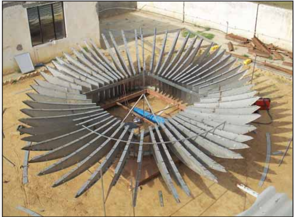
The structural frame of the Lotus in the central pylon is made of 304 stainless steel
