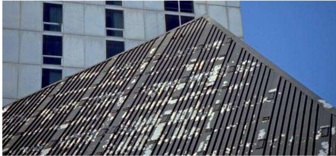
Peeling painted aluminum roof, 25 years
