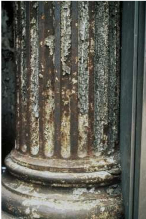
Peeling painted carbon steel
