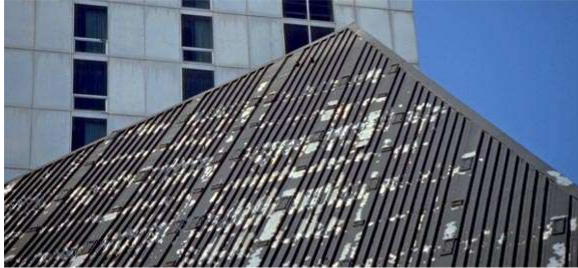
Peeling painted aluminum roof, 25 years
